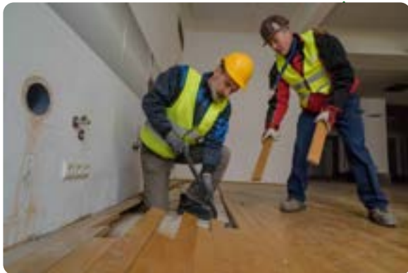
Removal of parquet flooring at MedUni Campus Mariannengasse, Vienna (2019-2020, Bundesimmobiliengesellschaft) © Harald A. Jahn
